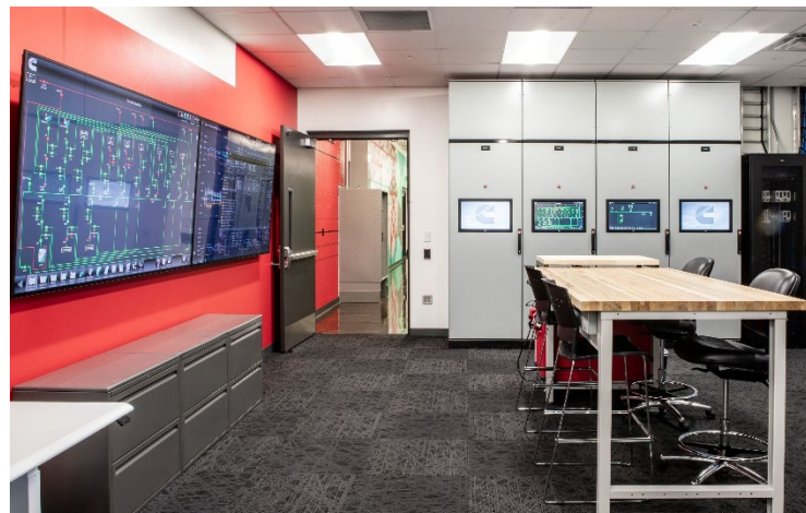
Control Room & Office Space
